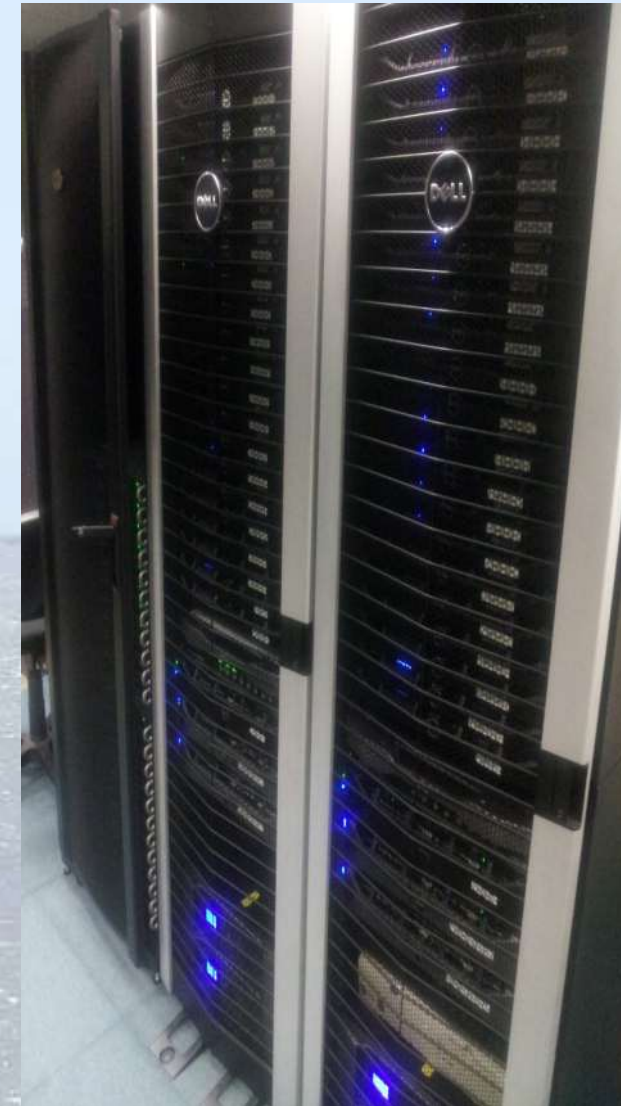
The pretty half of the server room
